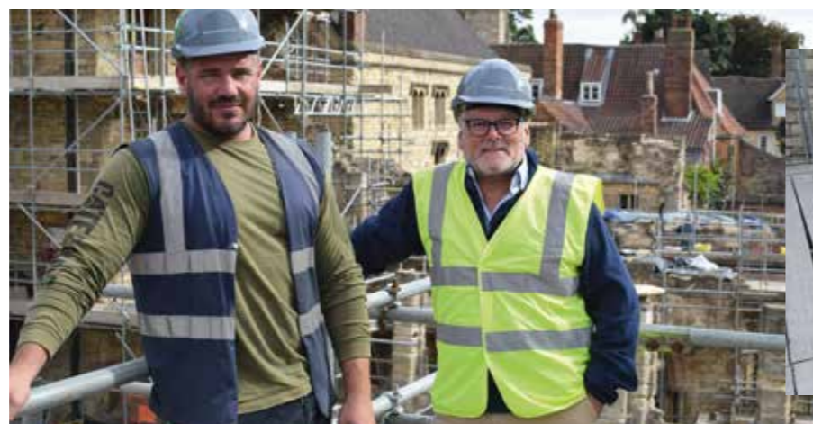
From Messenger, Jamie 'Paddy' Lilley (left), the Site Manager, and Fred Markland, Heritage & Conservation Senior Building Surveyor, showed NSS around the site.
