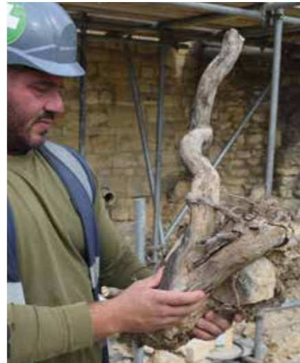
Site Manager Paddy Lilley with one of more than 1,000 plant roots removed from the walls.
